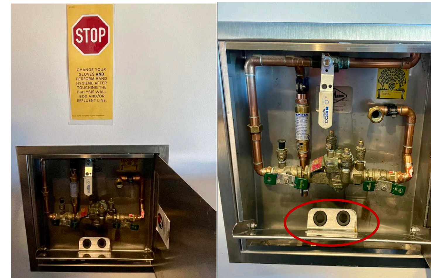
Figure 4. Reconfigured dialysis wall box with double grommets.
