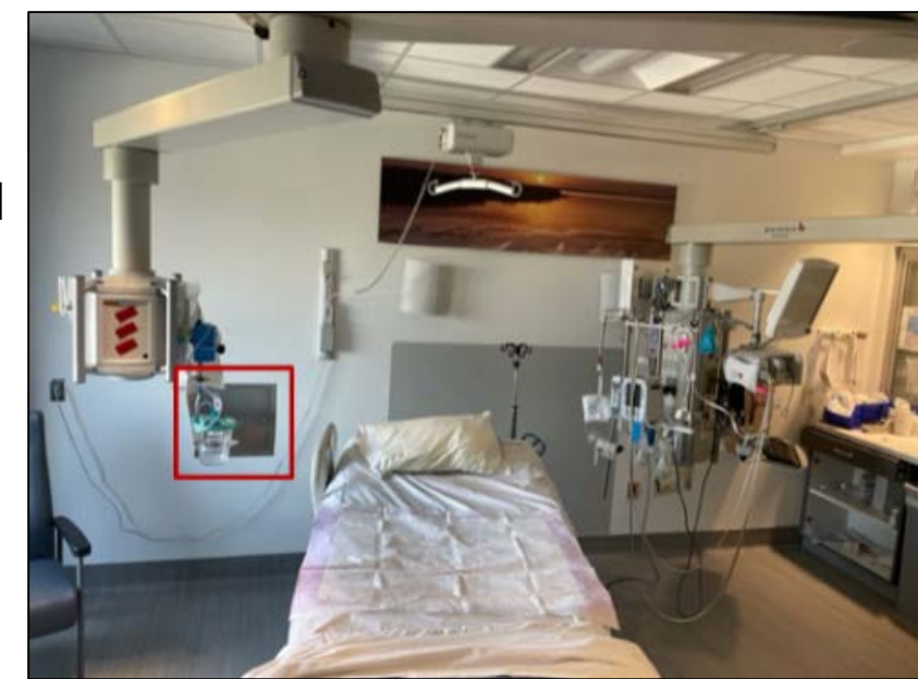
Figure 1. ICU room. Dialysis wall boxes (red box) are frames recessed into the wall that house drainage lines to discard effluent (i.e. spent dialysate or waste) into the sanitary sewer system.
