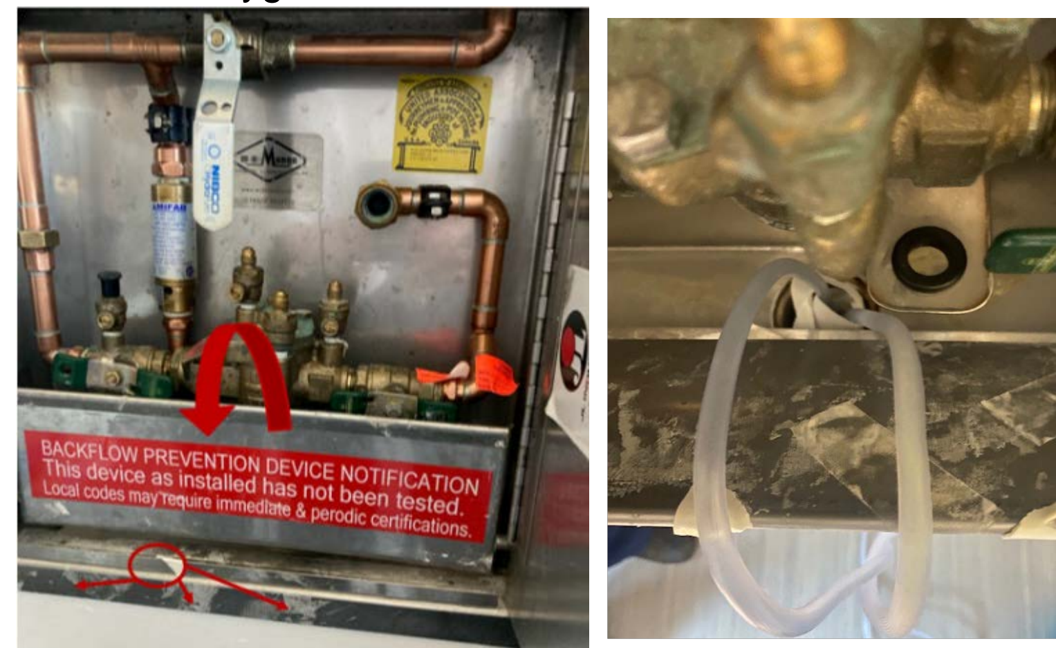
Figure 3. (left) Dialysis wall box with door opened and visible tape and adhesive residue and fold-down drip tray up. (right) Top view of wall box with effluent tubing threaded down drain and secured by staff with tape.
